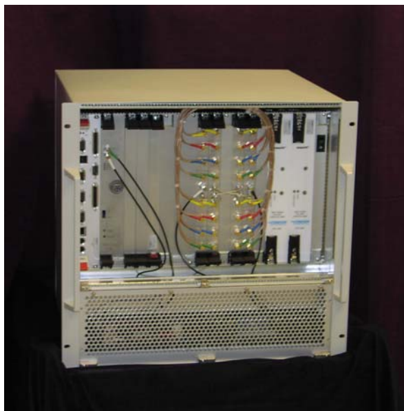
Figure 4-5 SGR Test-Bed Rack Mounted Configuration
